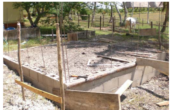
Initial foundation courses with reinforcing steel and earth fill. Forms for entry-apron underway.
